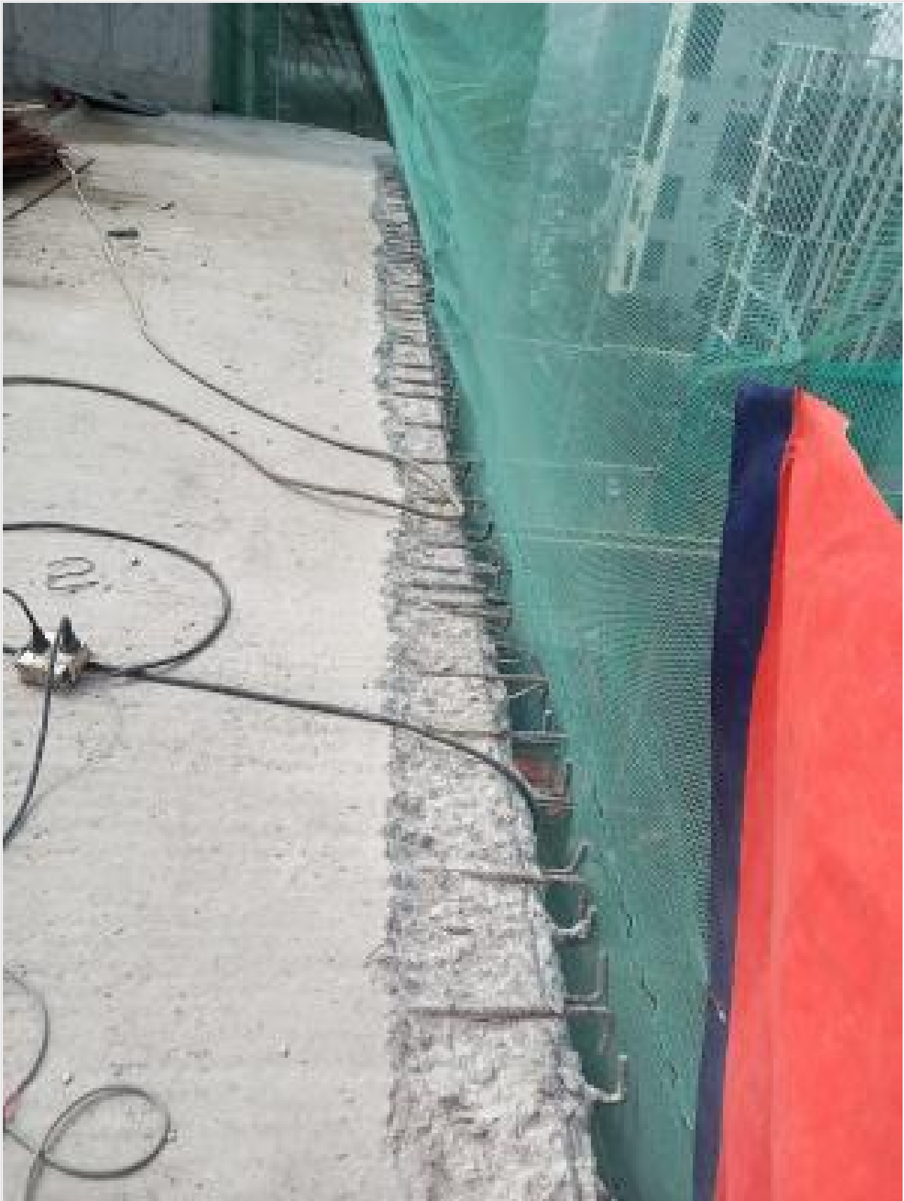
L-17-Slab chpping on 30-03-23
