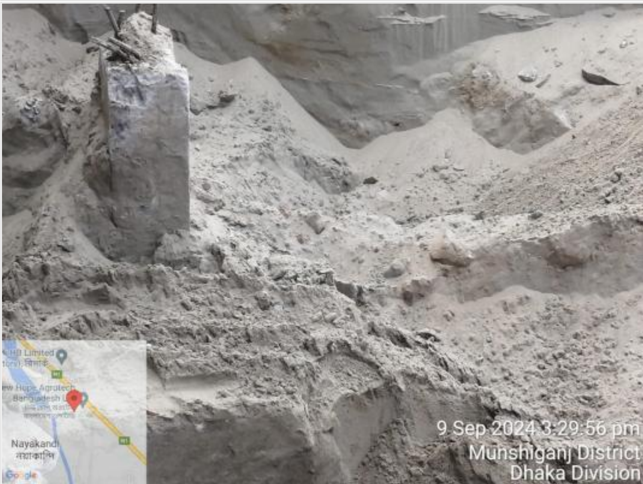
Old short column found durring excavatio on 09-09-24
