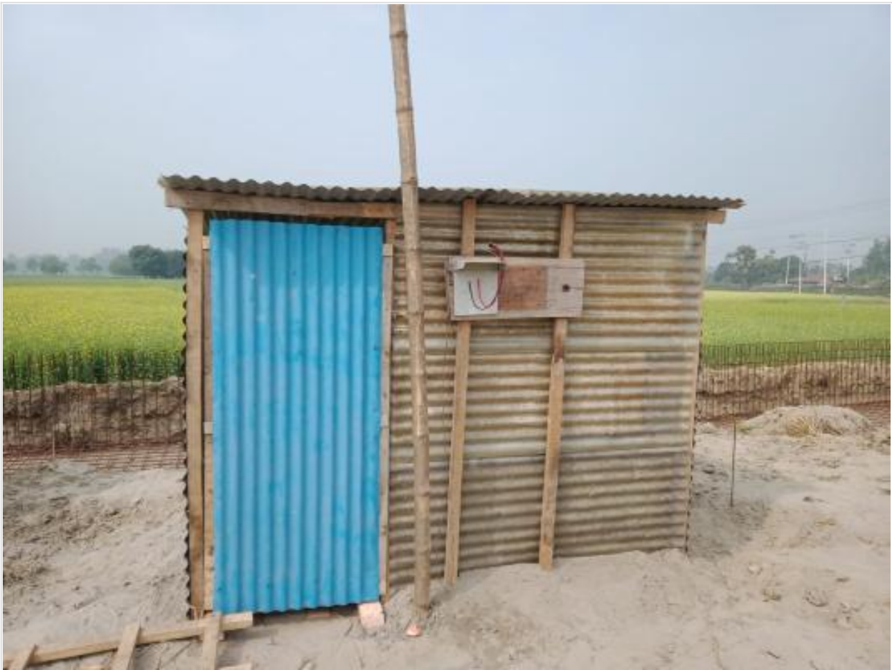
Electrical DB Setting on 31-01-23
