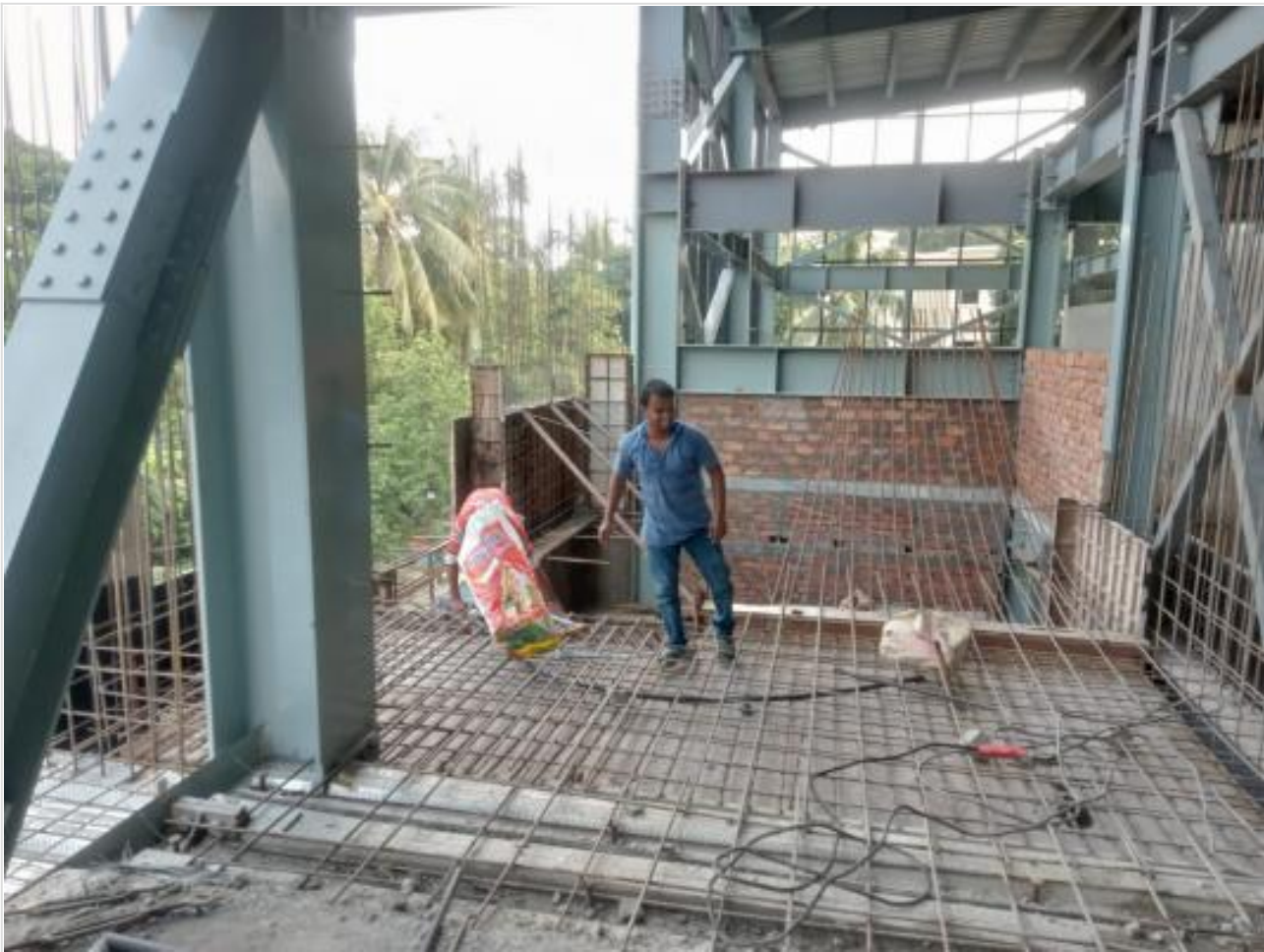
Stair rod binding on 03-09-21
