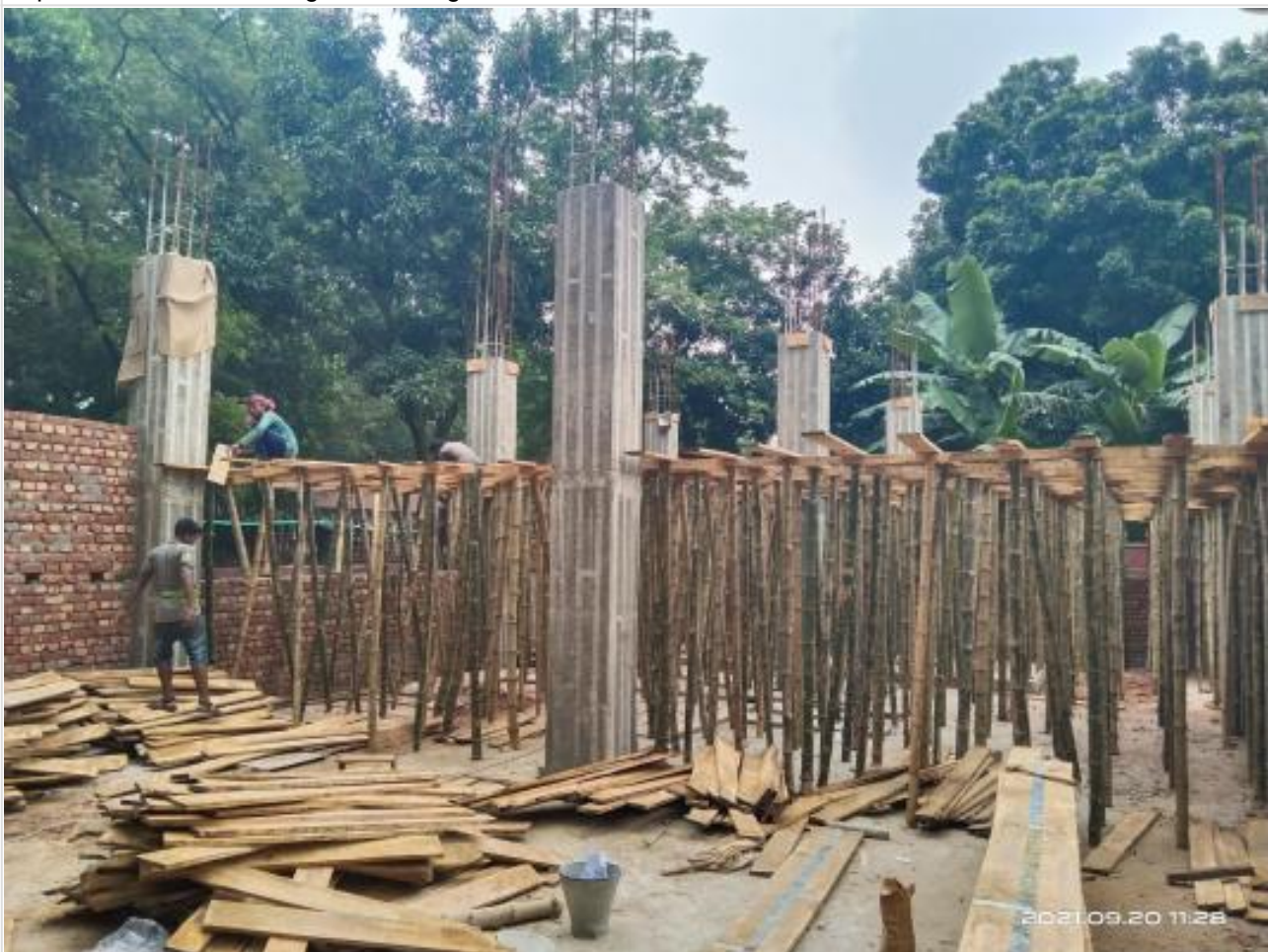
Sub-Station and Generator room staging f on 20-09-21
