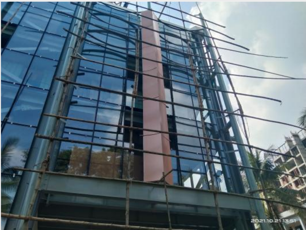
ACP fitting on 21-10-21
