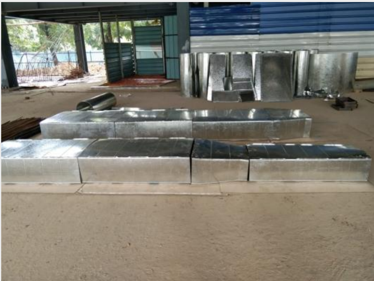
AC Duct on 11-05-21
