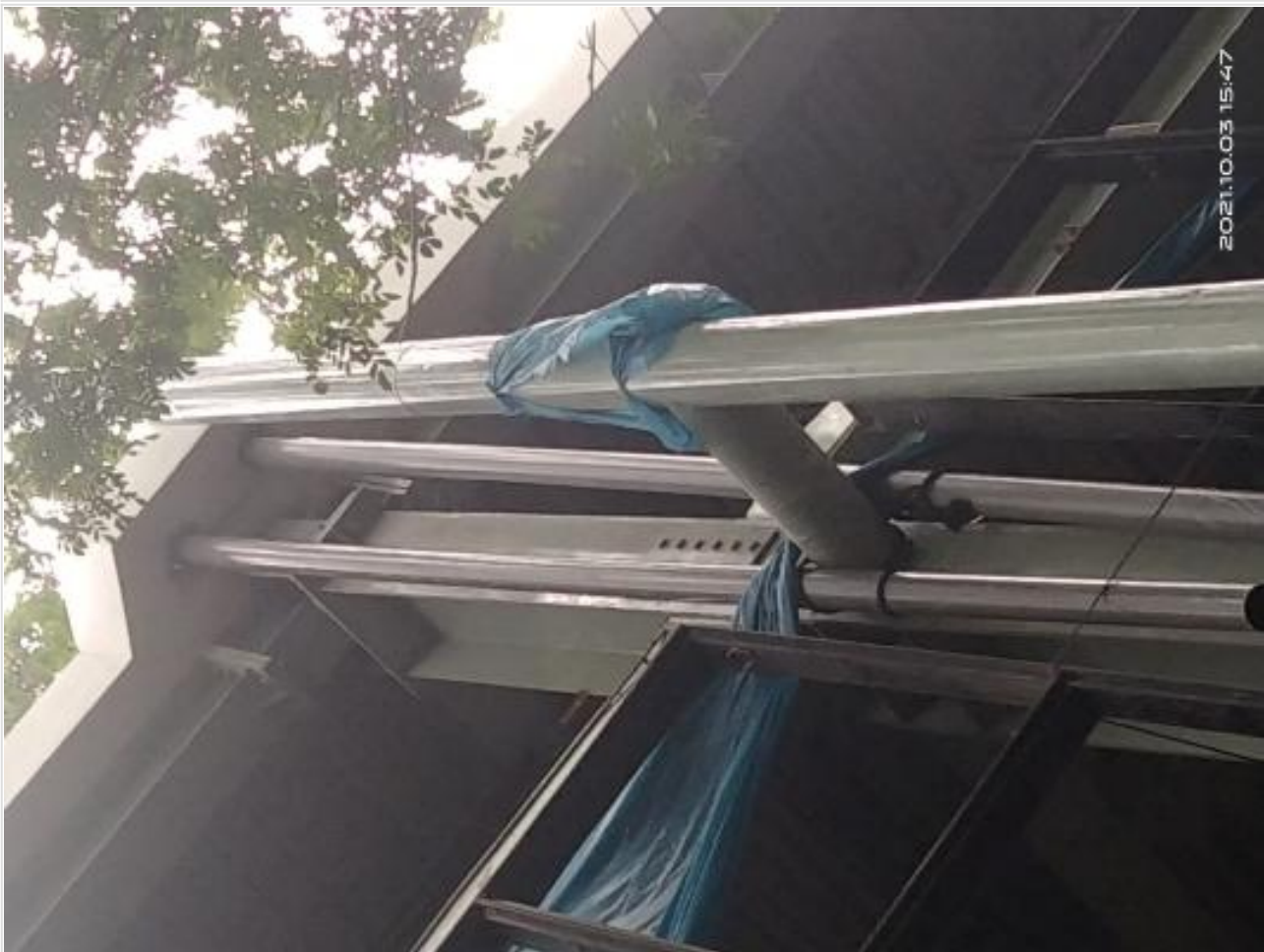
Rain water down pipe fittings on 03-10-21
