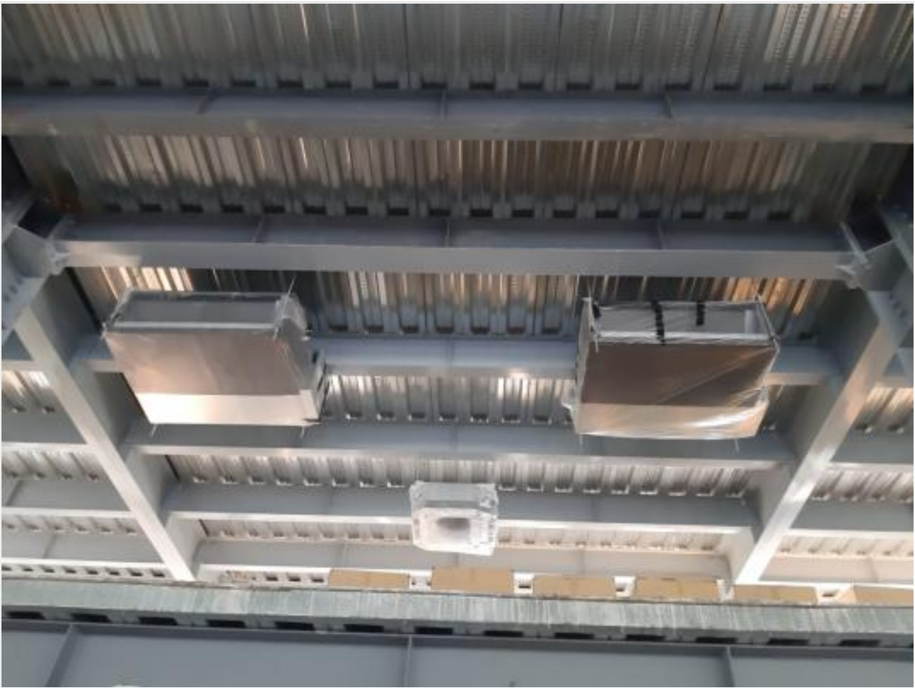
AC Indoor Unit Hanging on 09-05-21
