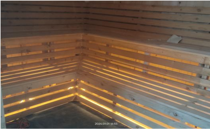
L-11-Steam-Suana-Wooden Wall-Lighting on 01-01-24
