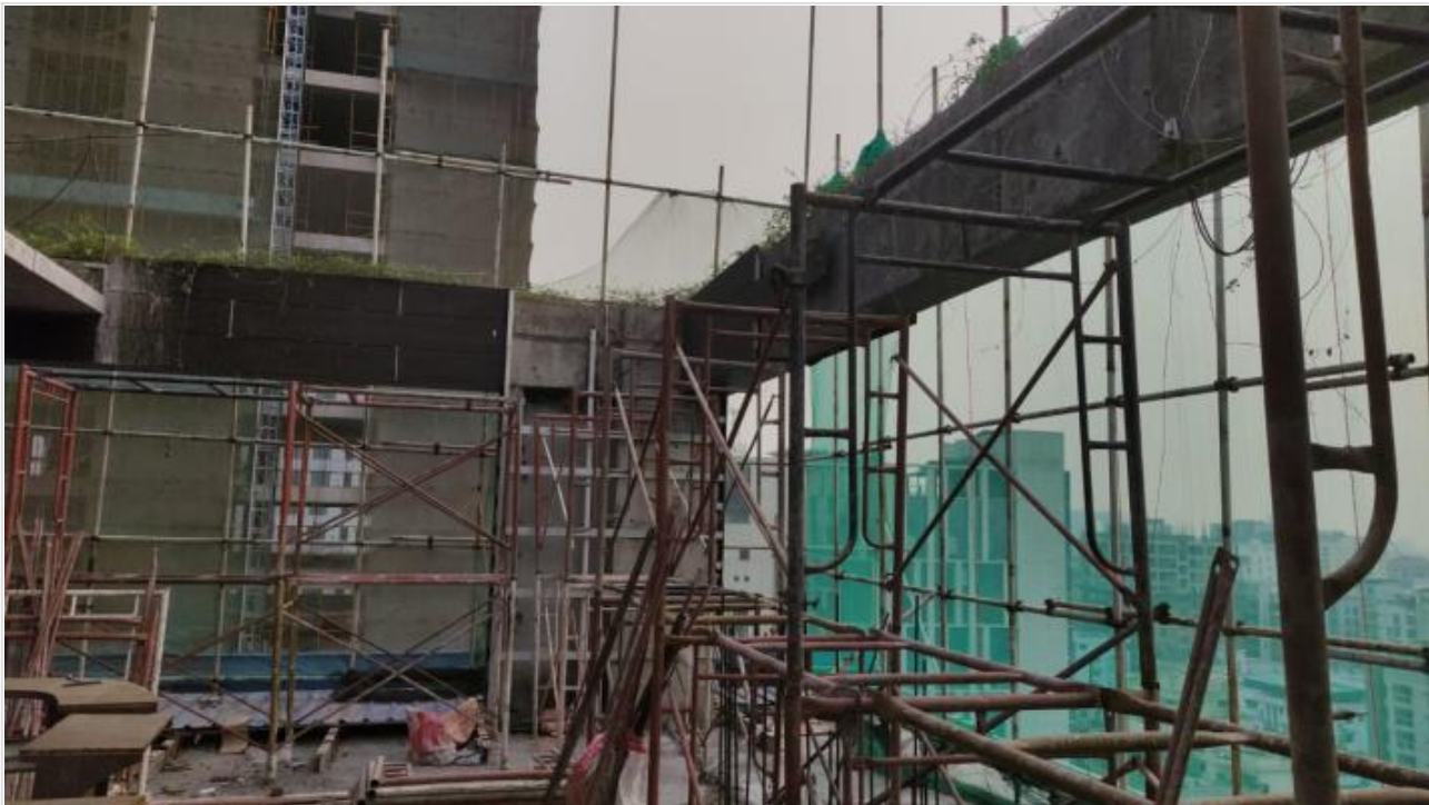
L-16-Safety installation on 18-03-23
