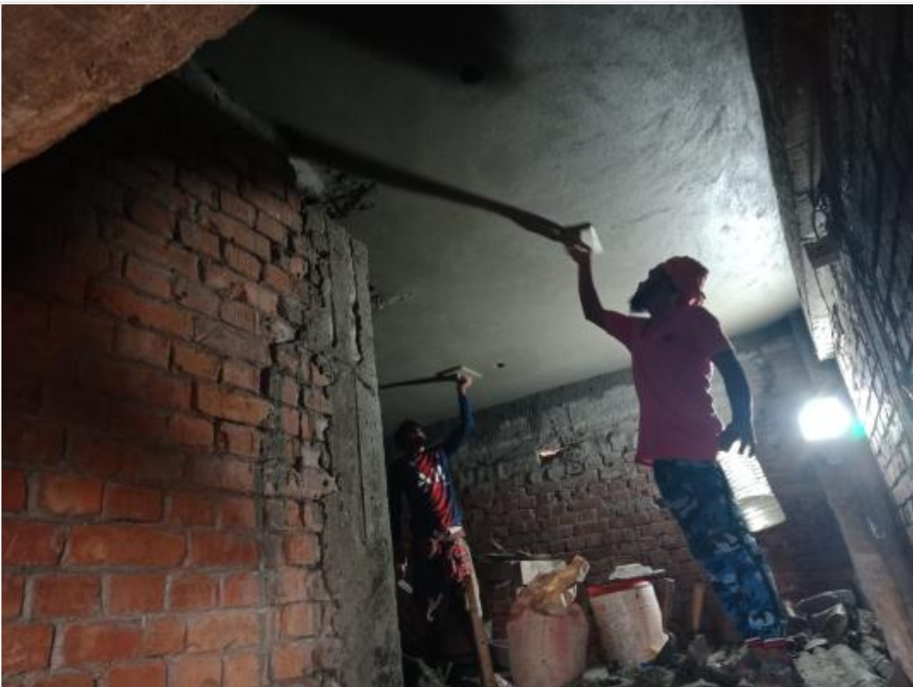
Dorm. Bldg. Ceiling Plaster on 01-11-23
