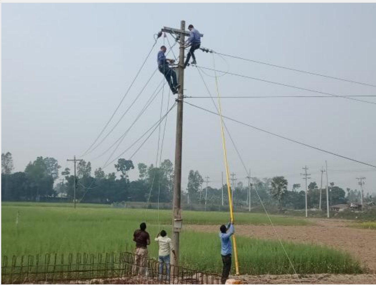
Electricity Connection on 06-02-23
